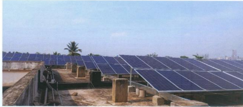
Solar PV Modules installed at rooftop of college
